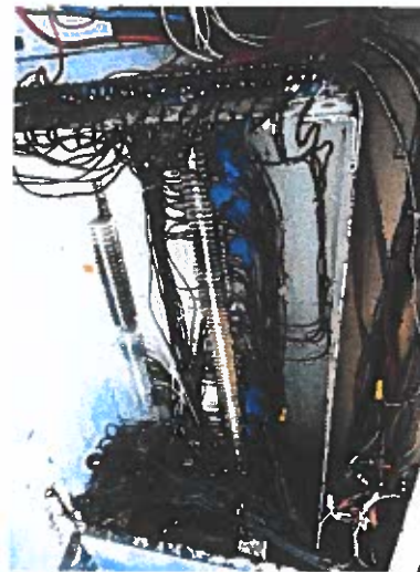
Photograph 6: North lock control panel 2 of 2
