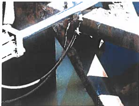
Photograph 15: South lock exterior conduit failure with exposed wiring
