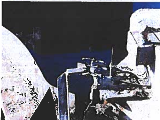
Photograph 3: North lock position limit switches
