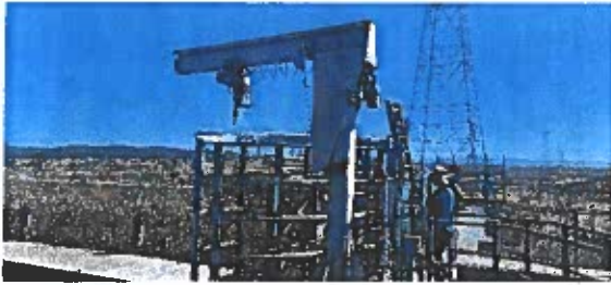
Photograph 11: Inoperable service crane at south lock
