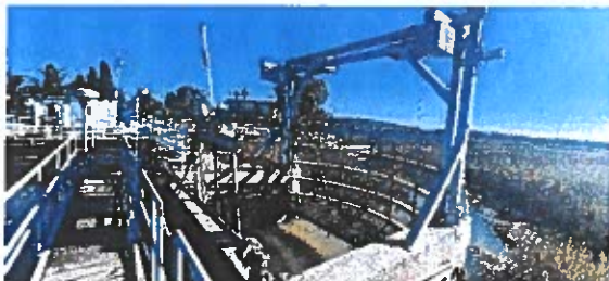
Photograph 22: Spillway gate with large strainer
