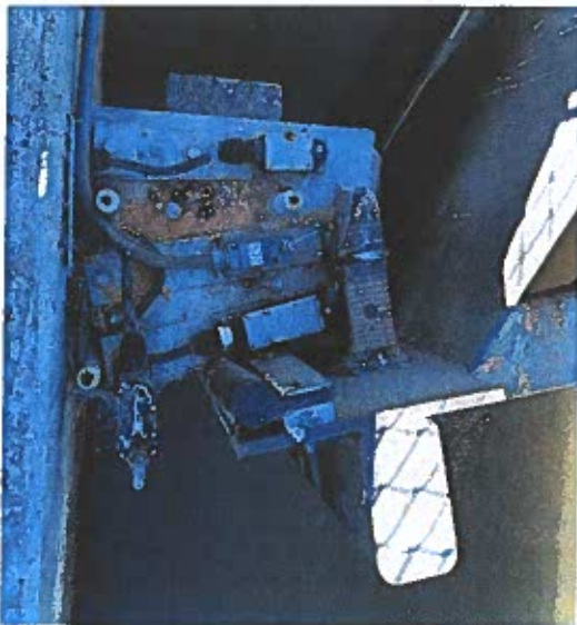
Photograph 13: Gate position limit switches on south lock with multiple switches inoperable and abandoned
